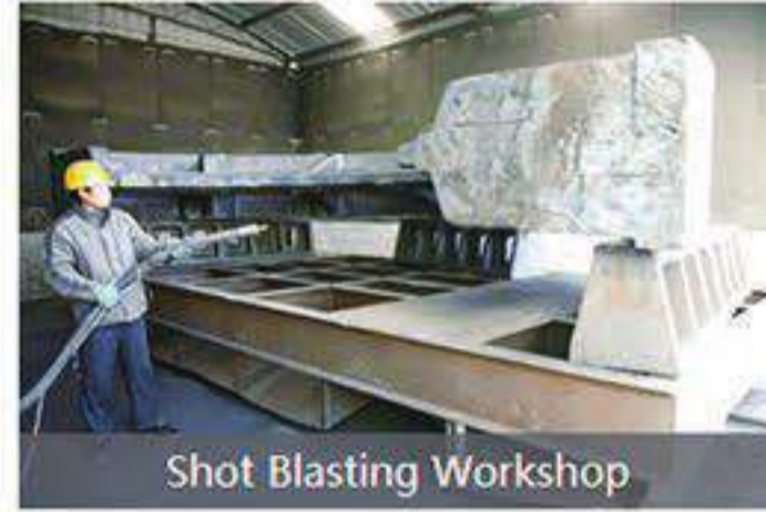
Shot Blasting Workshop
